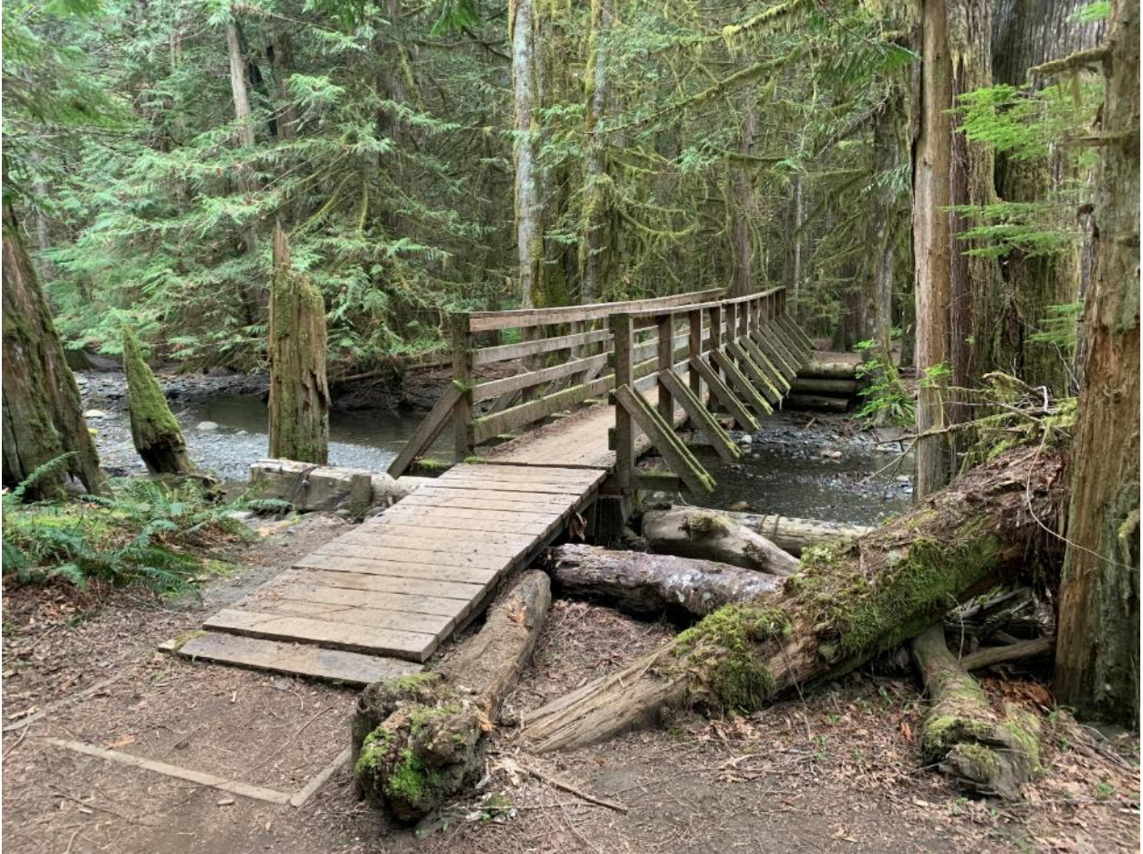
Figure 19. Bridge over Perseverance Creek requiring replacement.
