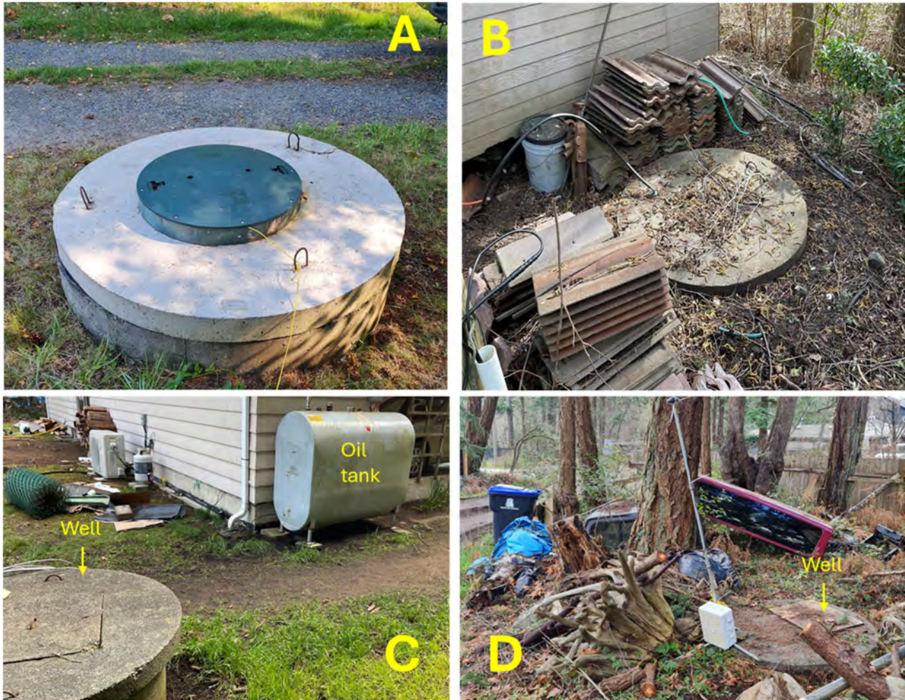
Figure 19: Observations of shallow, dug wells. A. Dug well with >0.3 m casing stickup above ground and sealed cap/cover is better protected from contaminants. B. Dug well with edge of casing at or below ground surface and gaps in the cover. When water from irrigation or rain runs off the site, muddy water and animal waste enter the well, causing bacterial contamination. C.-D. Sanitary area within 3 m radius around well must be kept free of foreign matter. Contaminants including septic fields/tanks, and fuel storage should be kept a minimum of 30 m from well.
